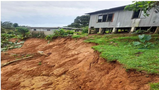
Figure 13q: Landslide at Vataleka in Wailoku. Source: National Disaster Management Office.
